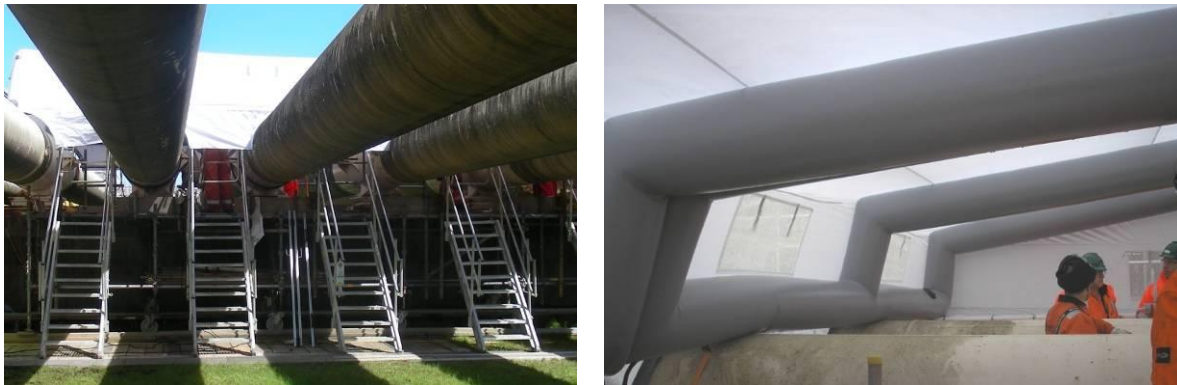
Figure 10. Smart access options: movable scaffolding on rails (after removal of stairs) and inflatable weather protection.
