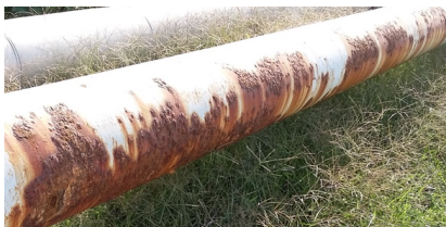
External Surface Corrosion
