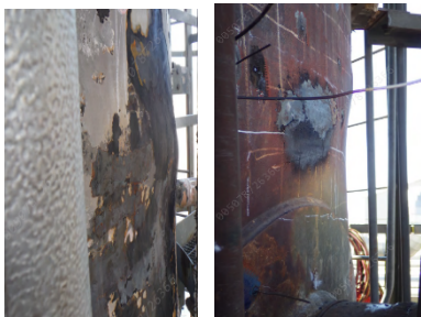
Figure-2 Distortion in a vertical vessel resulted from improper application of local PWHT [2]
