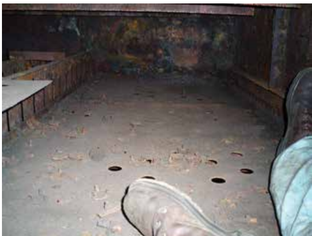
▲ Figure 9. Examine loose valves and the empty holes to determine what displaced the valves.
