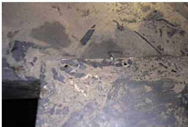
▲ Figure 19. Missing bolting hardware reduces the mechanical integrity of the tray, and is typically caused by vibration and/or loose installation.
