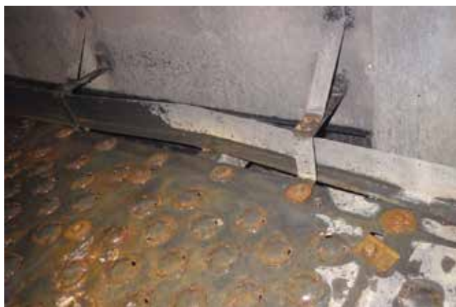
▲ Figure 15. This weir has been displaced and pushed away from under its retaining washers. Tower liquid can then bypass the weir through the gap under the weir.
