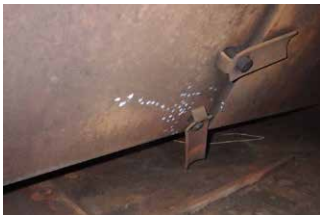
▲ Figure 16. This downcomer clip is bent from overtightening and has come loose, reducing the integrity of the attachment.
