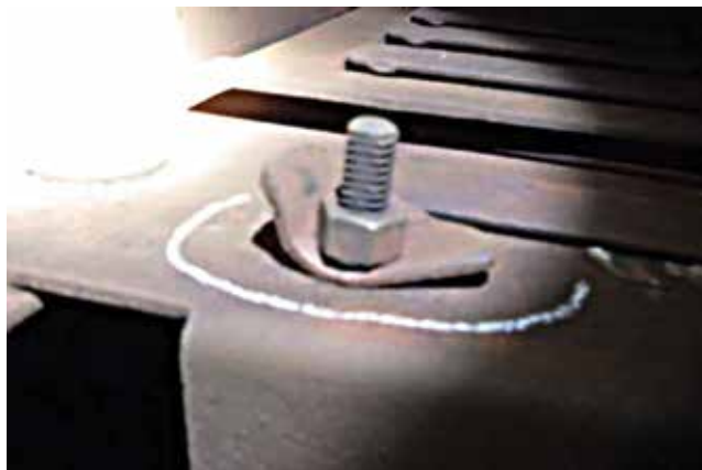
▲ Figure 11. Manway clips with a permanent bend must be replaced, preferably with 3/16-in.-thick clips.
