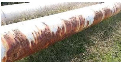
External Surface Corrosion
